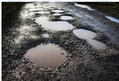
Fig -1: conditions of roads with potholes.
