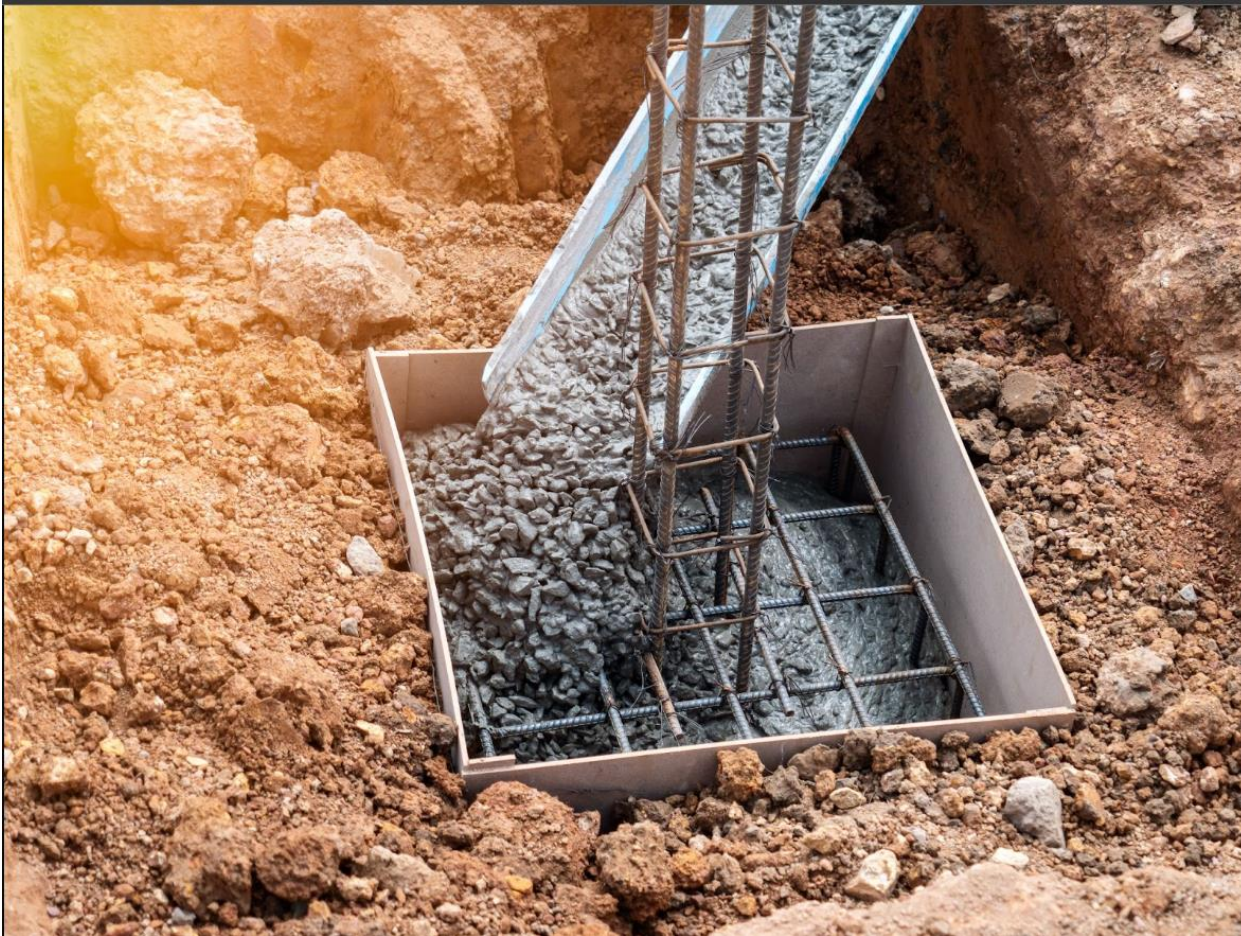
Fig.2: Solid Foundations- Pouring Concrete Columns for Strength and Stability (Image courtesy: what-is-a-footing-in-construction )
