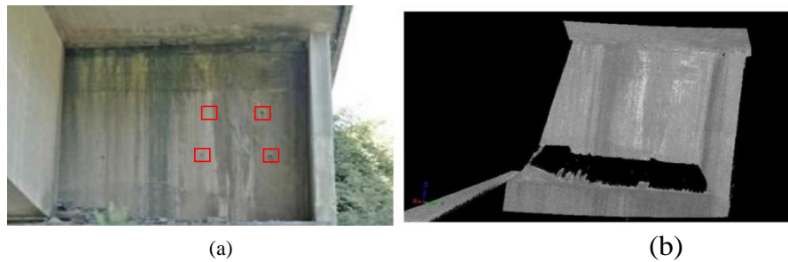
Fig. 14. Geometric survey with laser scanning of the wall of the North abutment, East side (station #3): (a) photo of the analyzed area and reference points; (b) point cloud.
