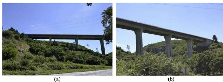
Fig. 10. Viaduct of IC2, over EN114, Rio Maior, Portugal: (a) North part; (b) South part.
