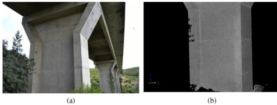
Fig. 13. Geometric survey with laser scanning of the North face of column P1 (station #2): (a) photo of the analyzed area; (b) point cloud.
