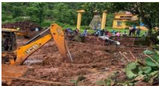
Fig1 : landslide in Posare village in July 2021
